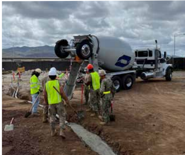
Service Members lay the foundation for the Special Olympics Hawai'i Health and Fitness Building and Play Court at the IRT construction site in Kapolei, Hawai'i.
