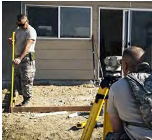
In FY 2020, IRT missions delivered $2.1 million in Civil Engineering value to communities across the United States.
